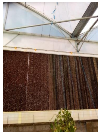
Fig. 5. Cooling pad wall
